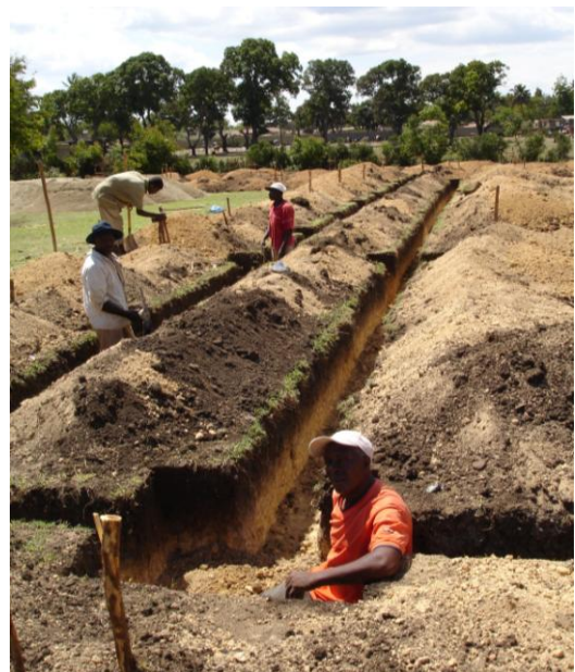
Trenches are being dug for the foundation of the Lycee Nationale school addition, the public secondary school in Pignon.
