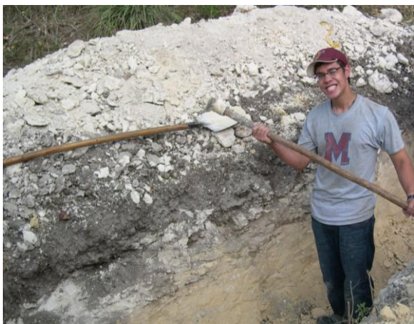
Haiti Outreach Intern Walter James digs out a lime soil mixture used to build a house.
